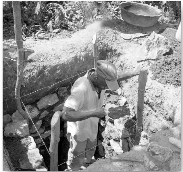
Jacques Jean, an ICC employee, not only supervises the latrine project, but also works side by side with local laborers.
